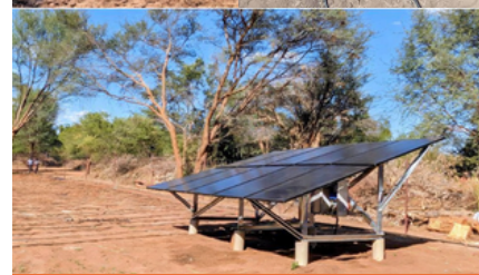
Solar-powered irrigation system installed under the S4CRPU Project in Kazungula
